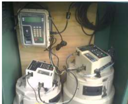
Figure 11. An example of the autosamplers used for wet weather water quality sampling. Two samplers were required for the samples analysed. This picture was taken at the Nunawading site.
